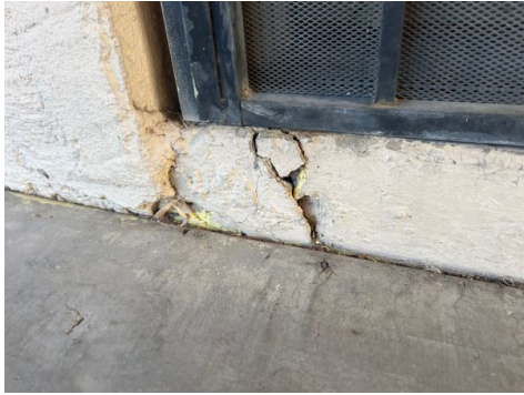
Below front door
